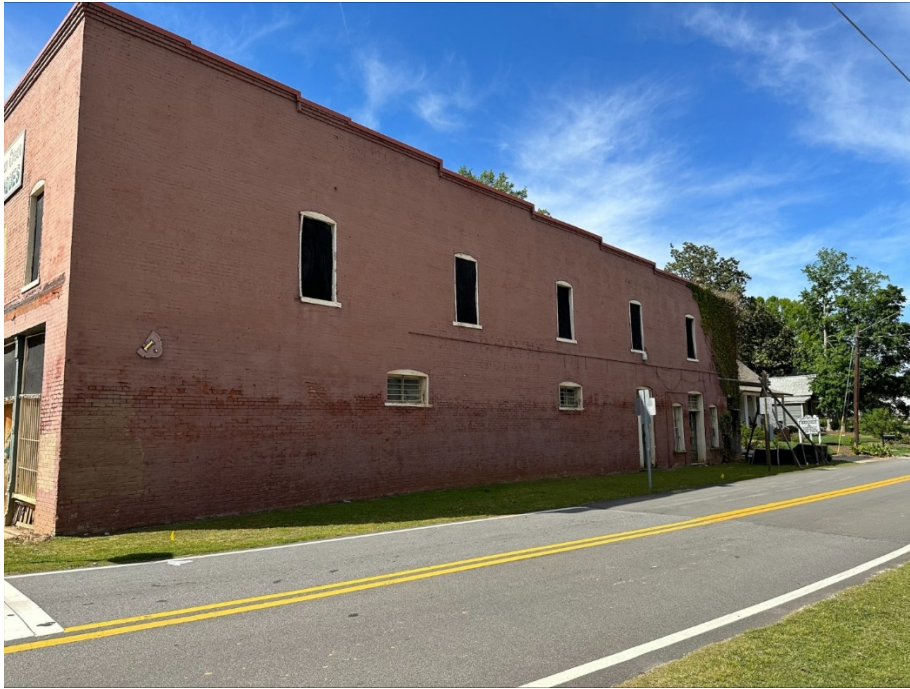
Photo showing mural wall facing Main Street, in its current condition, prior to renovation. A portion of the front of the building can be seen at the far left of the photo.
