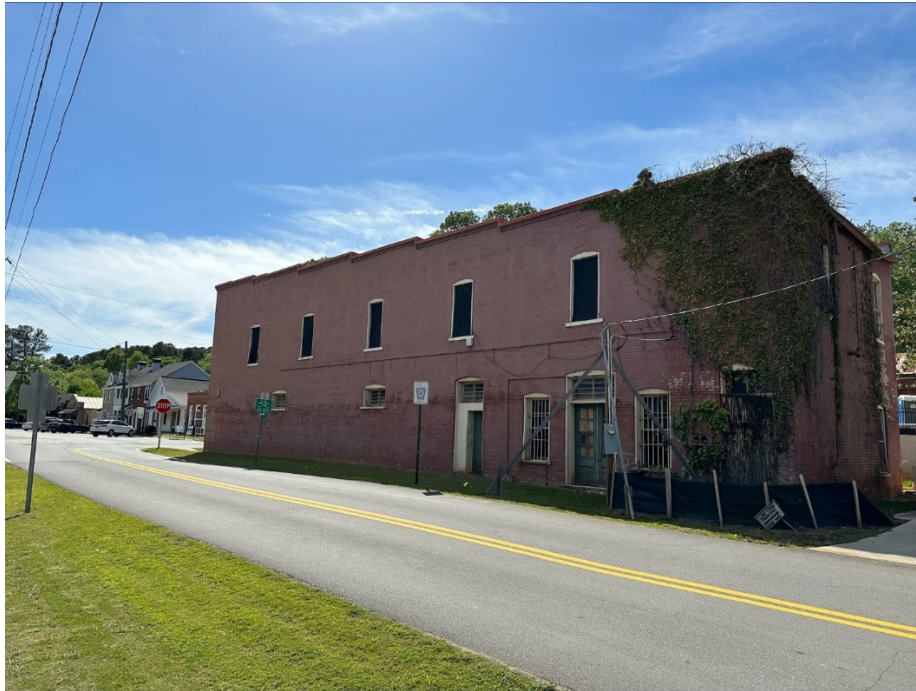
Photo of mural wall, in its current condition, prior to renovation, with view of businesses on the left side of the photo.
