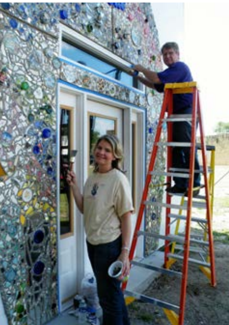
Volunteers install mosaic panels on the front of Bowl Plaza. Image courtesy Grassroots Art Center.
